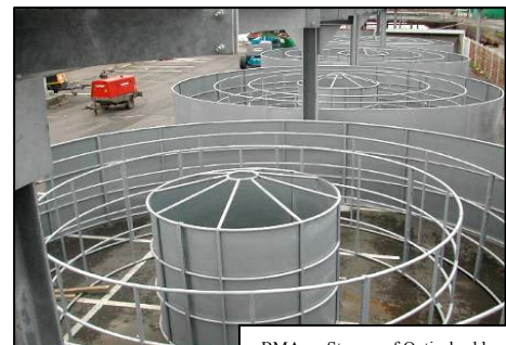
BMA Storage of Optical cables
